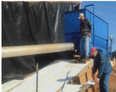
Hopper With Outlet Pipe Leading To Area Inlet
